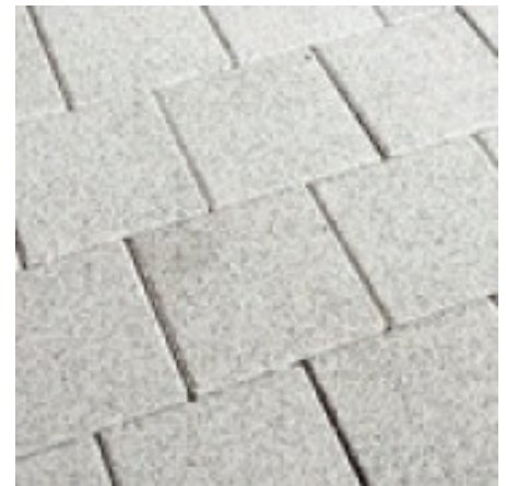
La Linia with CleanTop® after cleaning
